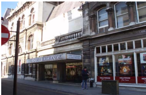
Corn Exchange, Ipswich - façade stone cleaning, restoration and roof repairs [c £900k project over 39 working weeks]
