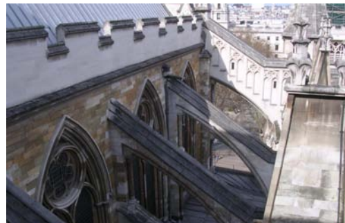
Westminster Abbey - repairs to the east aisle north transept roof [c £400k project over 38 working weeks]
